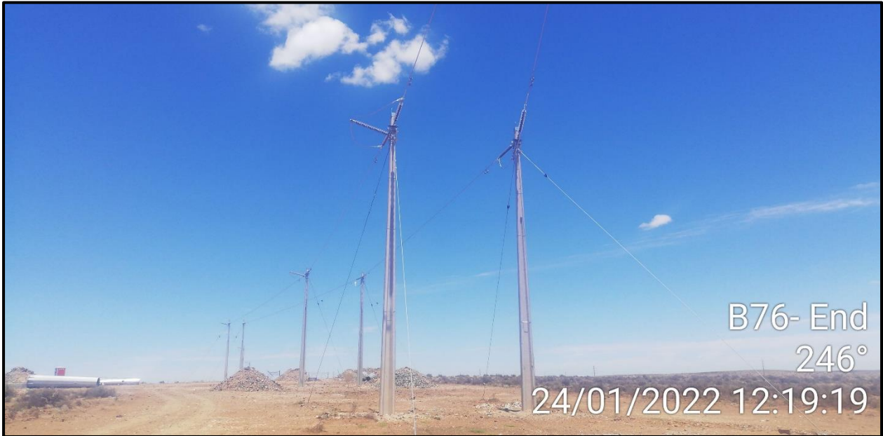
Photograph 3: illustrating the end point of the 4.5km 50kV Bypass powerline together with the surrounding infrastructure and surrounding environment.
